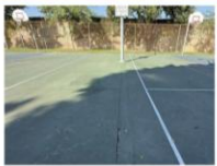
E. CRACKING SURFACING AT SPORTS COURTS
