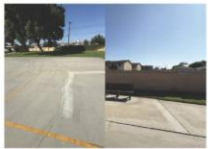
F. CRACKING CONCRETE AT SPORTS COURTS
