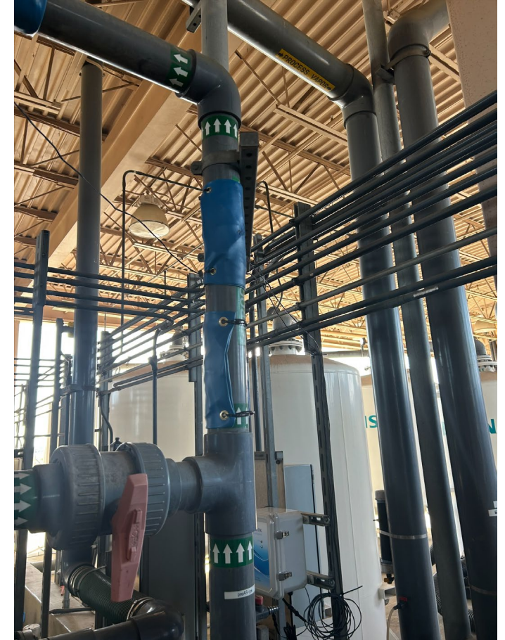
FlowMark Installed at Intake Lines Prior to Air Stripper in LOC
