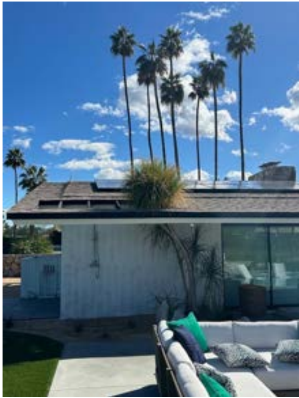
Northeast corner wall and roof opening, looking south
